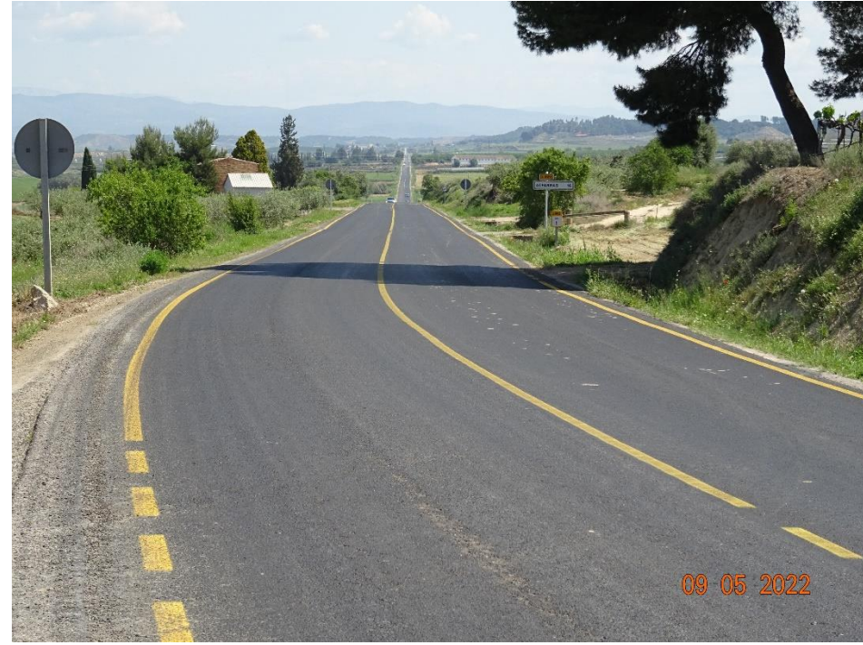
CIR Lane, fog seal and temporary striping, prior to HMA final seal
