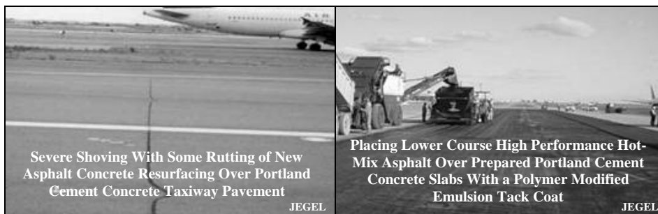
Photograph 6 Localized Severe Shoving of New Asphalt Concrete Resurfacings of Some Heavy Aircraft Traffic Areas at Pearson International Airport Has Required the Development of High Performance Hot-Mix Asphalts and Special Construction
